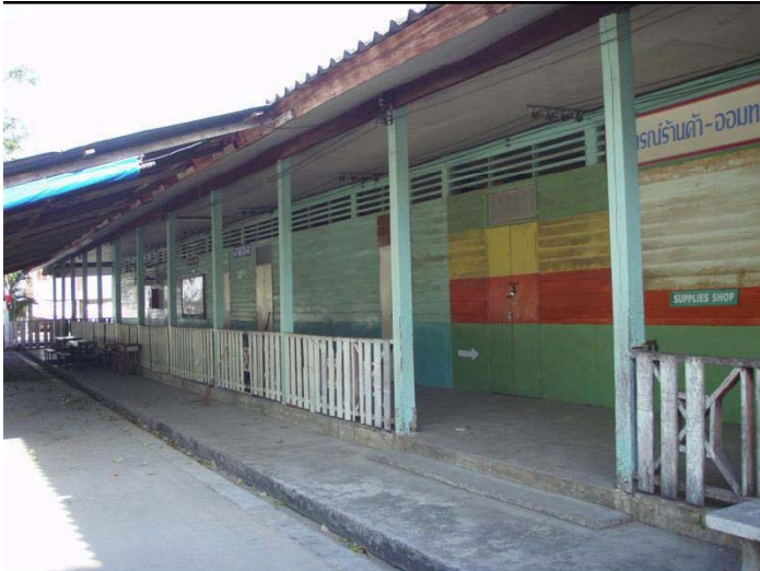
Outside of cafeteria needs painting Cafeteria and bathroom needs painting
